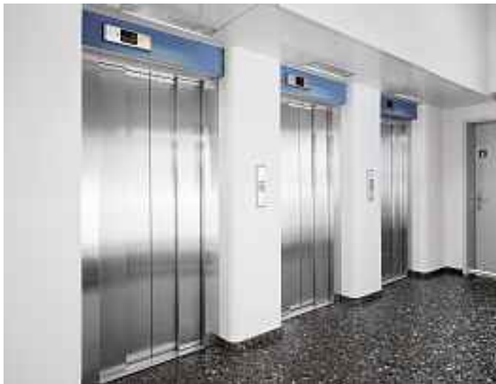
DO SEC car and landing doors
